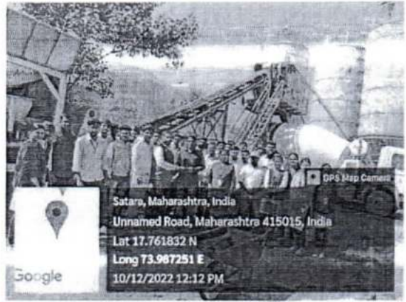
FIG.NO.2 RMC PLANT
